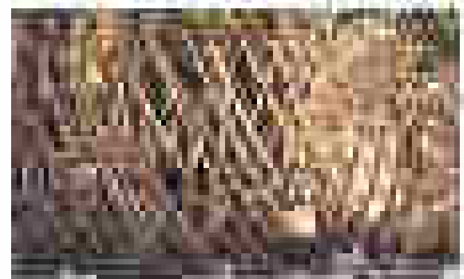
Figure 11: A photograph showing a close-up of a textured, possibly stone or concrete, surface with a vertical crack or crevice.
